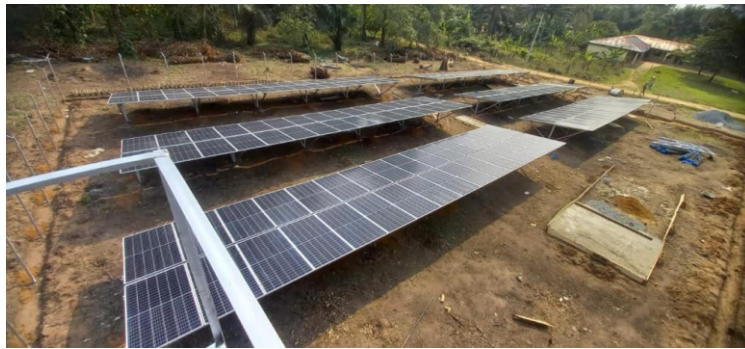
Construction of 50KW Solar mini power grid at Obadore, Odigbo Local Government, Ondo State.
